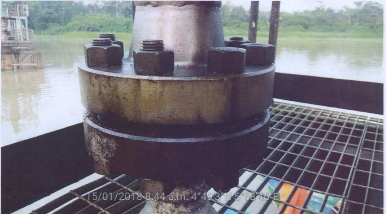
Fic C: Leak point
